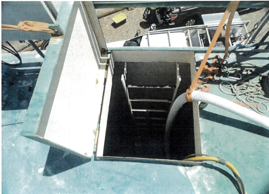
Looking into the tank from the roof hatch. Coatings have failed on the upper rung of the interior ladder and associated metal loss is present.
