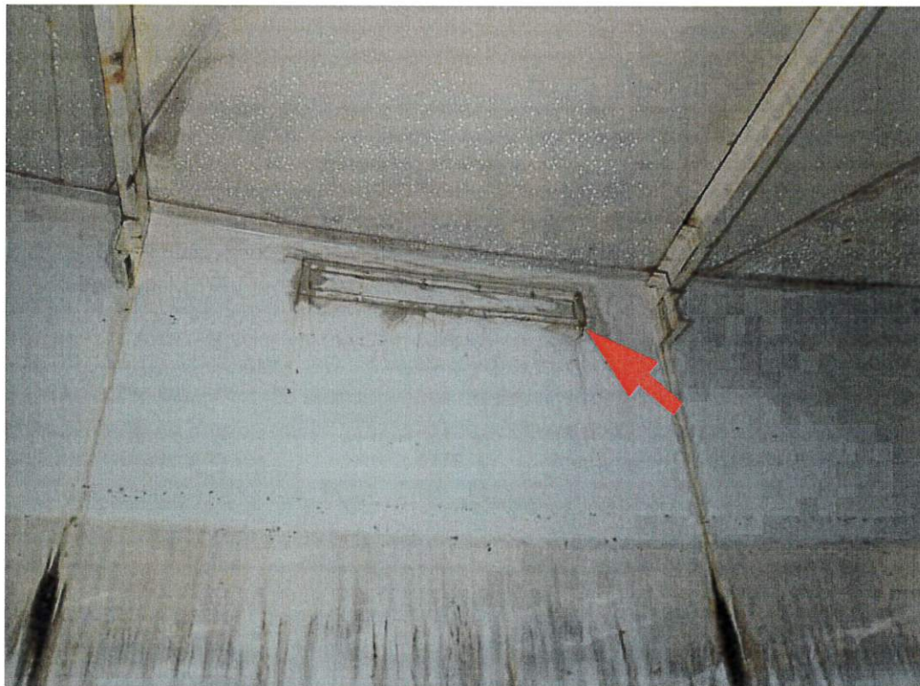
An additional view of the typical rafter and roof condition near the shell. The arrow shows a shell vent that has been welded closed. Scattered corrosion is present.
