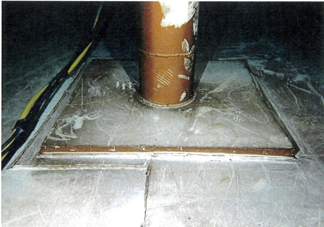
This photo shows the lower portion of the center column with welded base plate. Coatings are in good condition and no corrosion is present.
