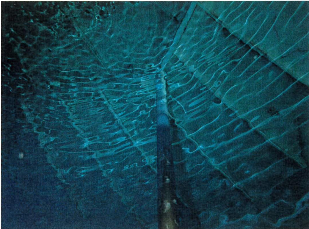
This is a typical view of an intermediate column looking upward near the surface. Some minor corrosion points are present.
