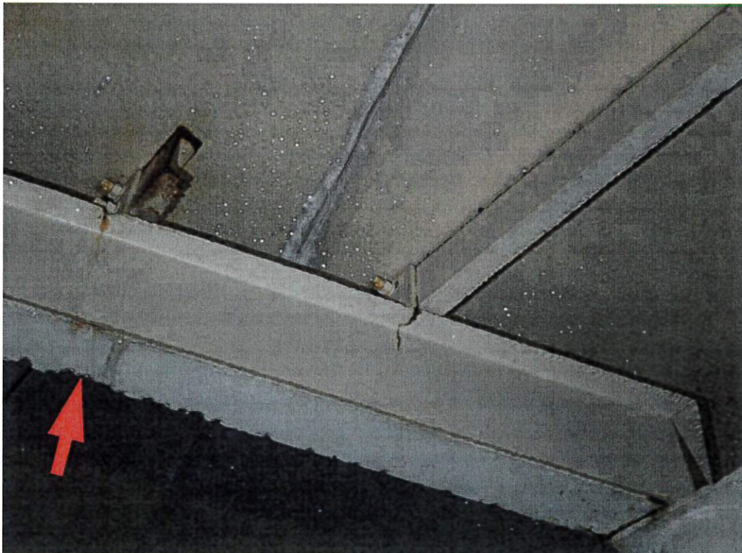
This photo shows a typical intermediate roof girder. Coatings are in good condition overall but corrosion staining is visible from inaccessible areas and significant metal loss is evident from prior to the application of this coating.
