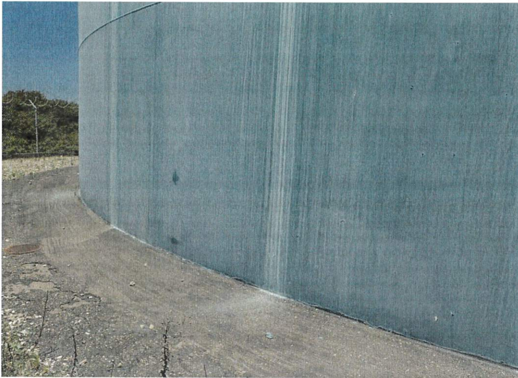
Lower shell and asphalt foundation. Chime is hidden beneath the asphalt pad.
