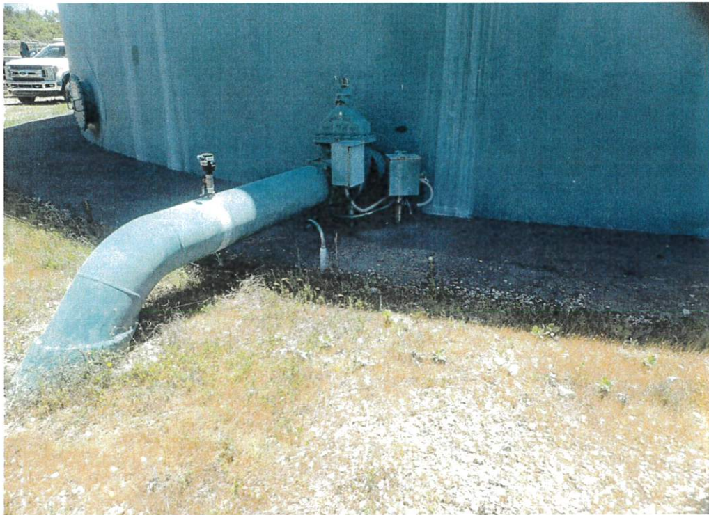
This view shows the inlet outlet piping penetrating the tank shell. This piping is more rigid than current seismic design standards allow
