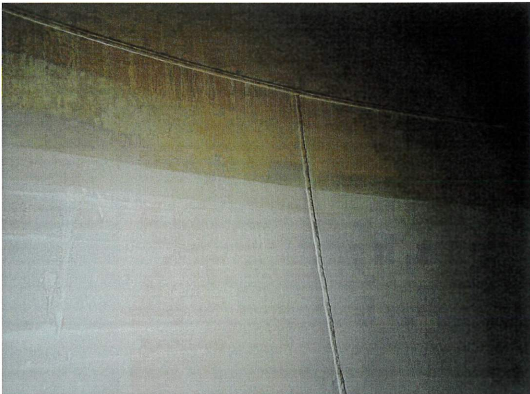
Interior shell in the submersion zone. This view shows a horizontal weld and vertical weld junction. The interior shell is in good condition.
