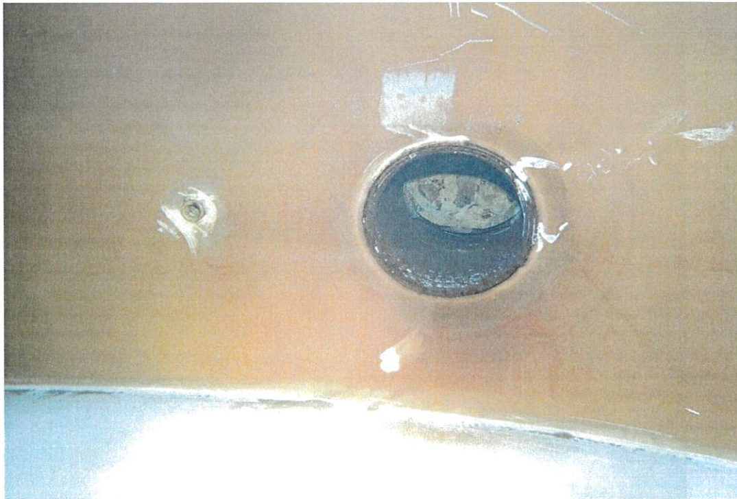
Shown above is an interior view of the inlet/ outlet piping penetration and sample tap. Coatings are in good condition.
