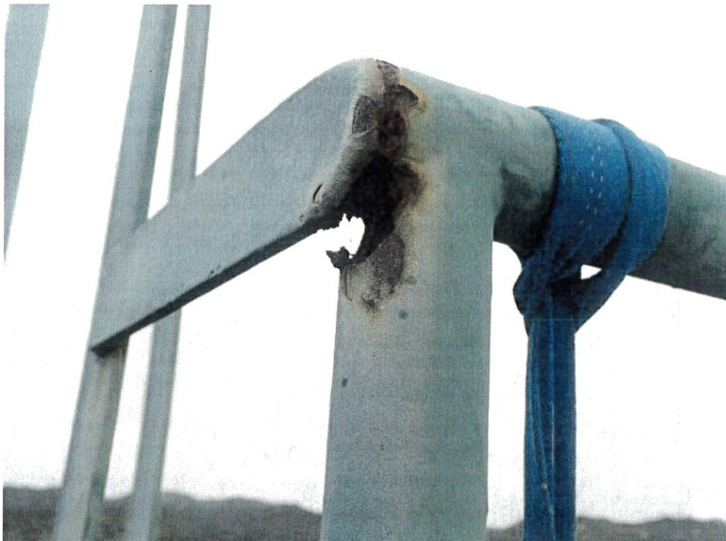
This photo of the roof guardrail on the south side of the ladder entry shows an example of the corrosion damage.
