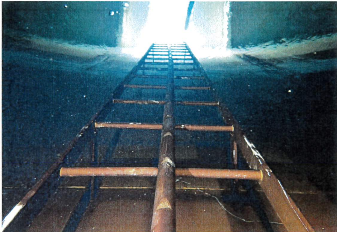
This view shows the interior ladder below the surface. Coatings are in good condition and protecting the steel.
