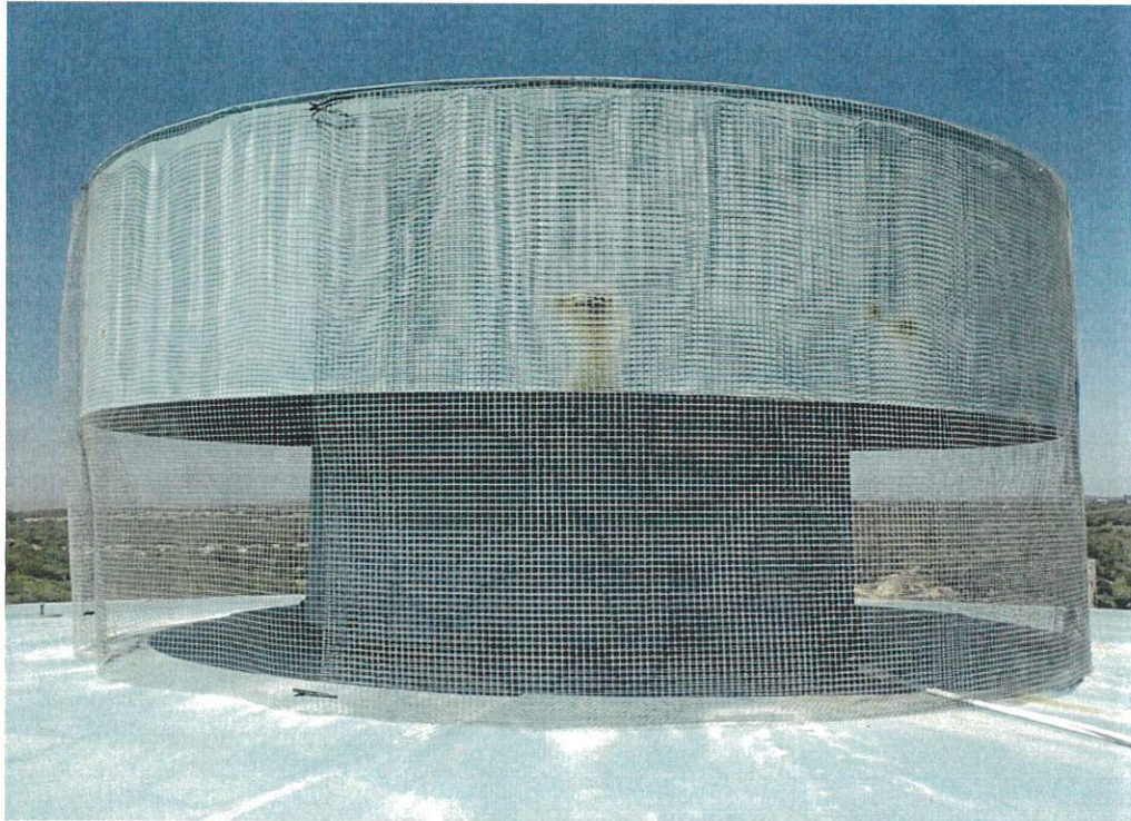
The roof vent consists of a steel cover over a steel riser pipe. The screens appear to be functional and "Bug proof".
