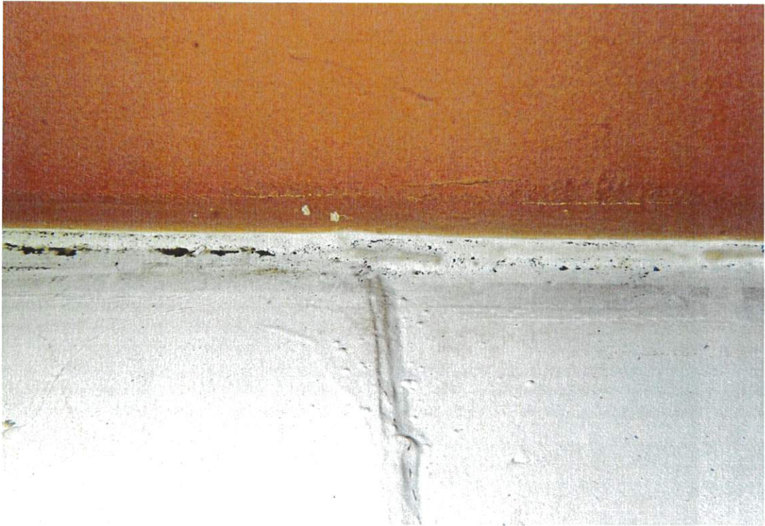
Lower shell and tank bottom with weld spatter.
