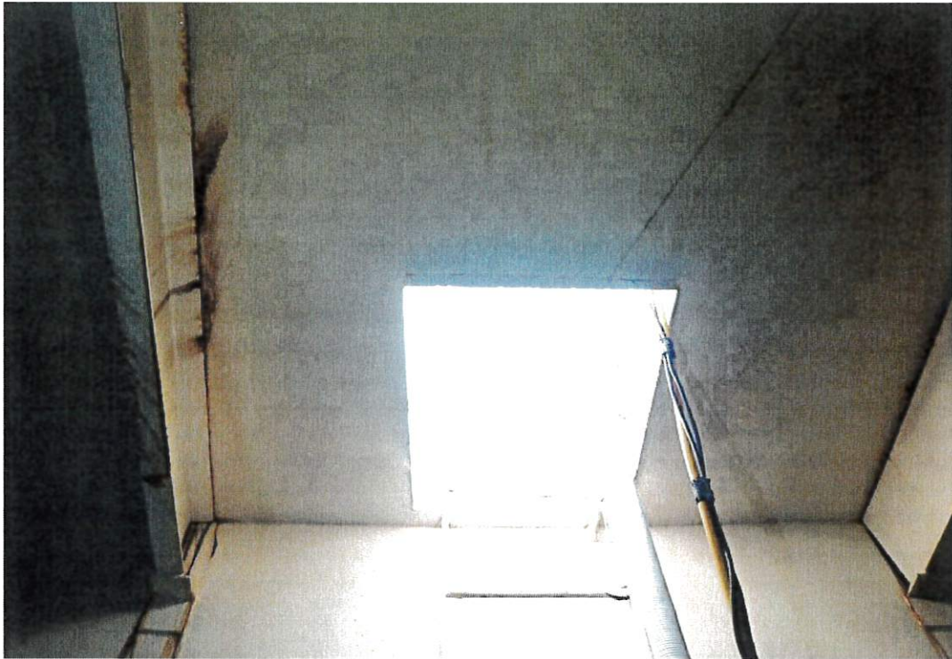
View of the roof hatch from the interior. Coatings have failed on the top rung of the ladder. Staining is present from rafter tops.
