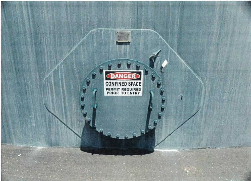
Shown above is a multi-bolt manway, lower shell, and tank nameplate. The manway itself is in fair condition with heavy chalking present.
