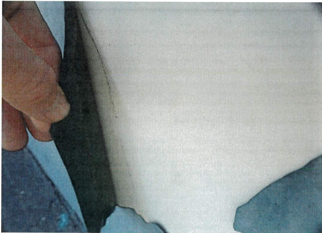
Severe inter-coat delamination is also present on the tank shell.
