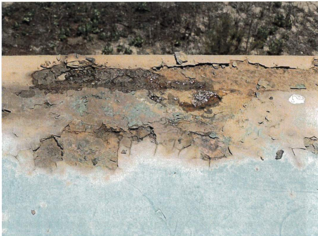
This closer view shows some of the serious corrosion at the roof's edge.
