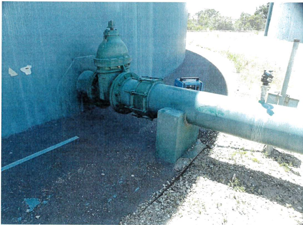
The inlet/outlet piping is more rigid than allowed by current design standards.
