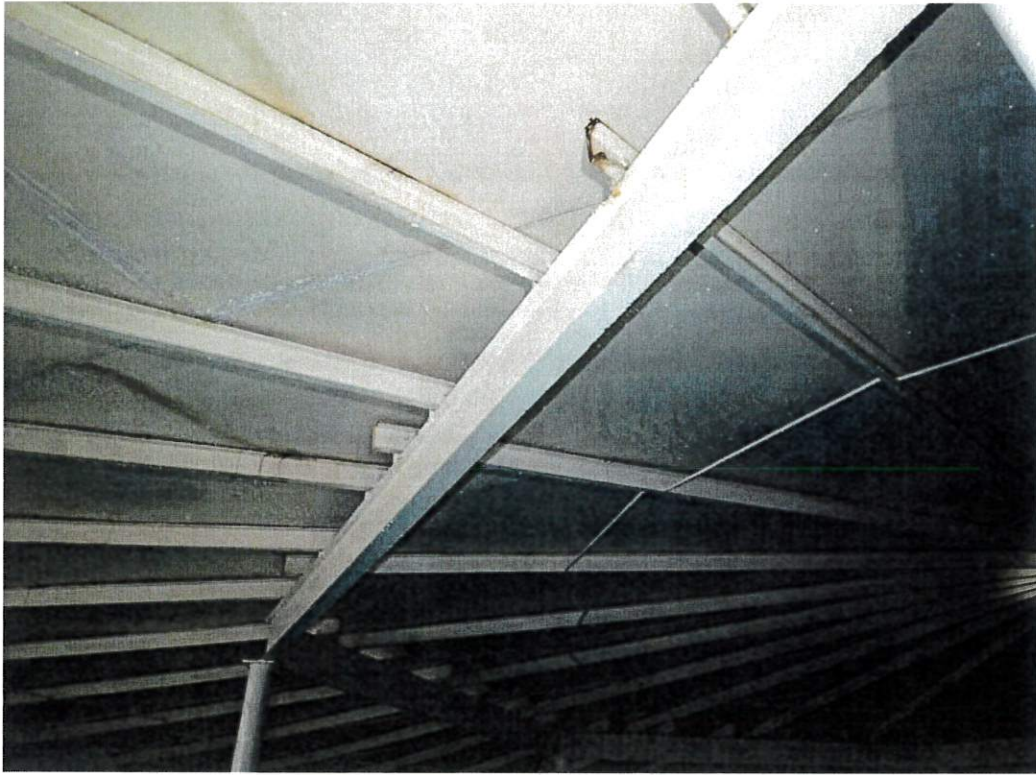
Interior roof plate, rafters, intermediate columns and girders. Typical broad view. Scattered corrosion locations are visible.
