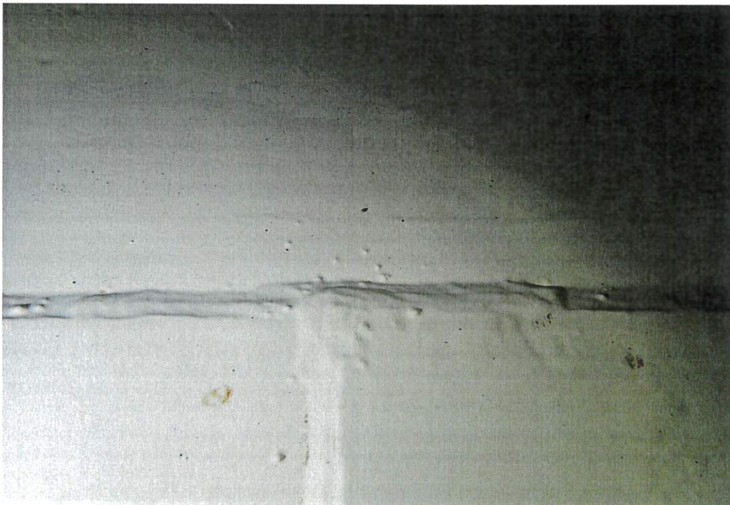
This photo is representative of the typical conditions found at plate joints on the tank bottom. Weld spatter is present underneath the coatings but rust is not present at this location.
