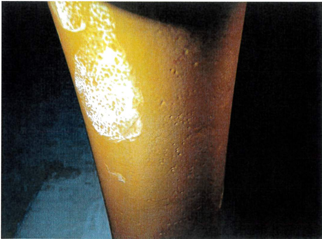
The photo of the center column represents the condition found on the lower surfaces.
