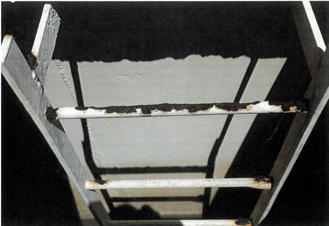
Coating failure and associated metal loss at the top of the interior ladder.
