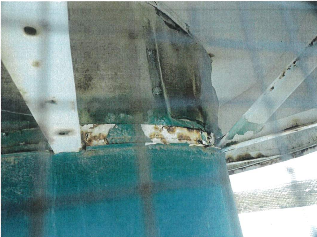
This view shows the vent screen, hardware and underside of the vent hood. It appears that the screen system may not be bug proof.
