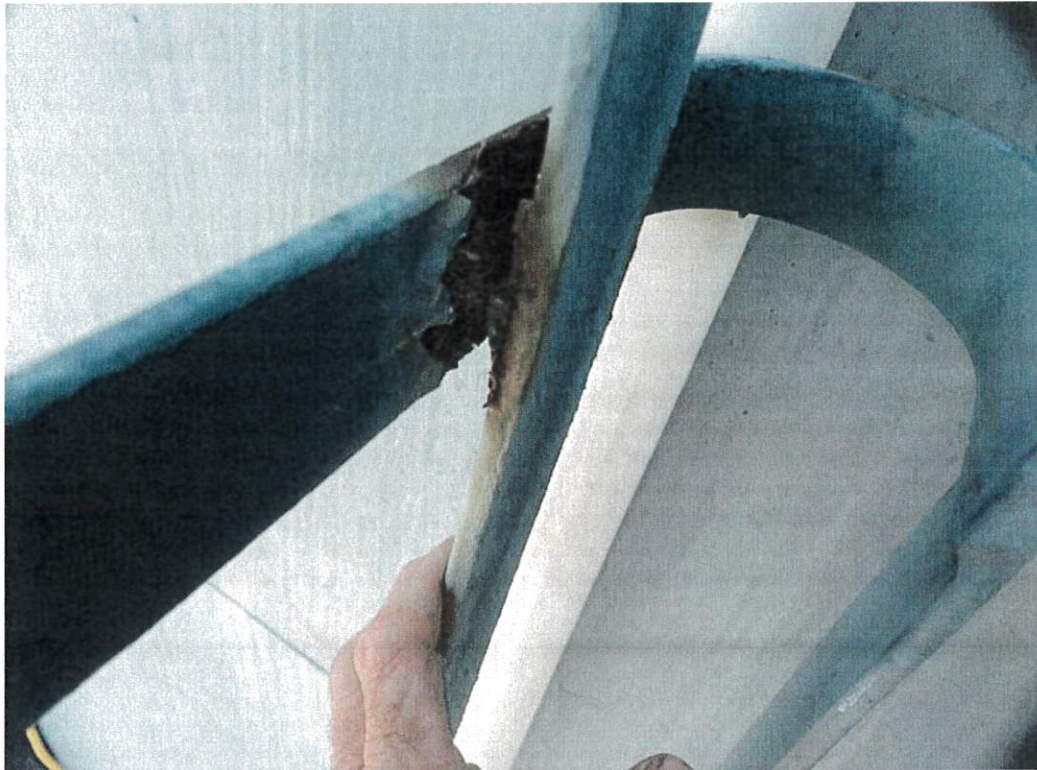
The photo above shows one of several locations on the ladder cage where welds are broken.
