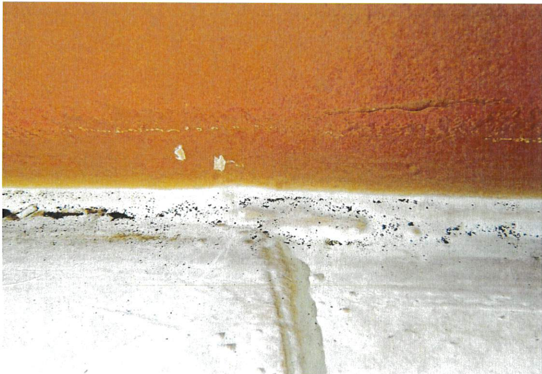
This photo provides a close view of the area shown in the top photo this page. Coatings are in good condition and protecting the steel.
