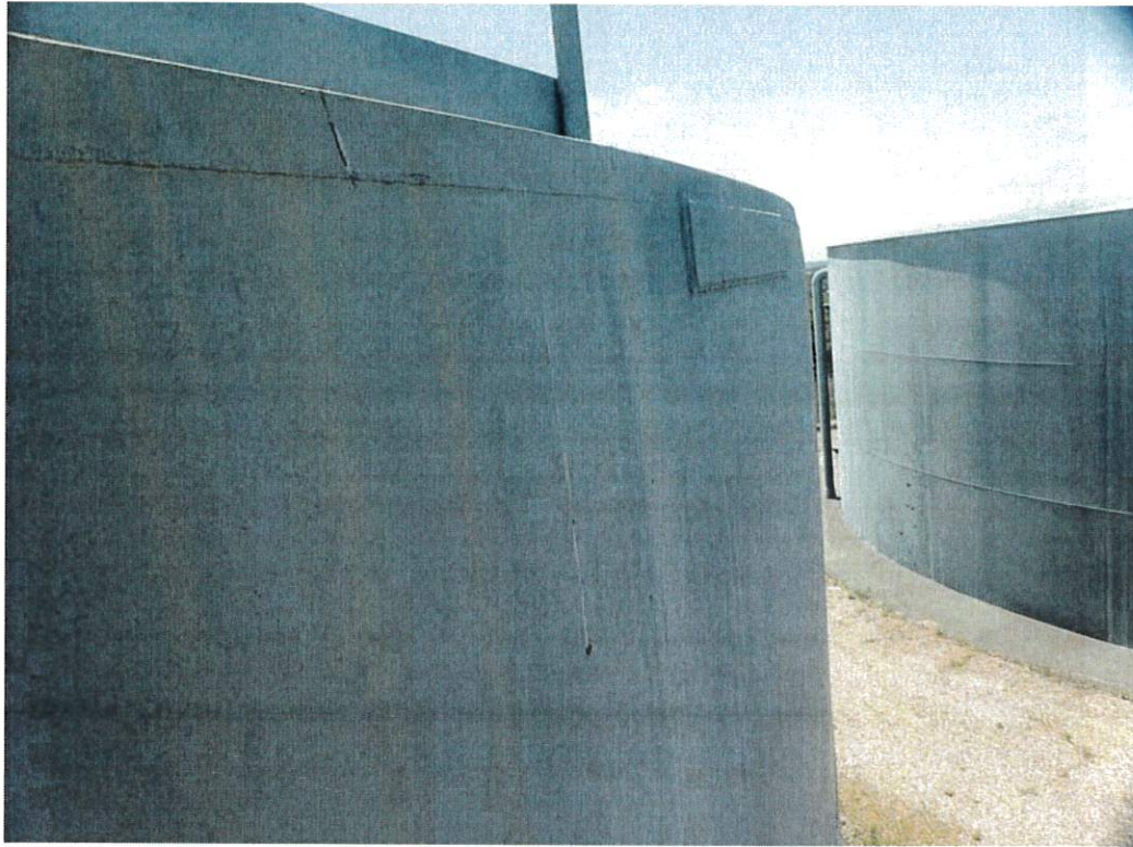
The upper shell and roof joint are shown in this photo. Significant chalking is present on the exterior. Chalking indicates that the coating is in poor condition due to aging and associated breakdown
