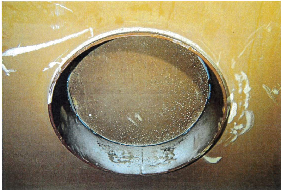
This view shows the interior of one of the two multi-bolt manways. Small blisters roughly 1/8" in diameter are scattered across the manway but coatings have not been broken.
