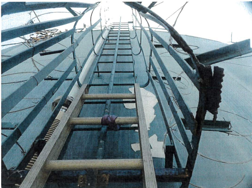
The downward swinging cage door, razor wire, lack of ladder to the ground and lack of ladder safety device to the ground may help prevent unauthorized access but they also increase hazards to authorized personnel.
