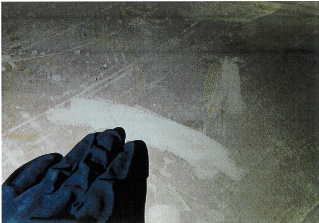
The middle section of the tank bottom (In front of the inlet/outlet) has a brown/ red stain that came off when rubbed by the divers glove.
