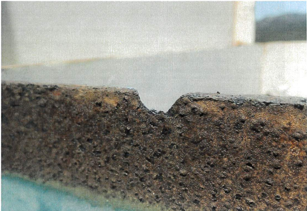
This photo shows the lip of the roof hatch. Severe corrosion is present.
