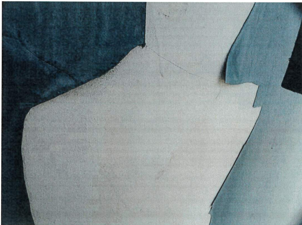
This close view shows an example of the green layer of paint peeling from the previous coating. Peeling is occurring in numerous locations on the exterior.
