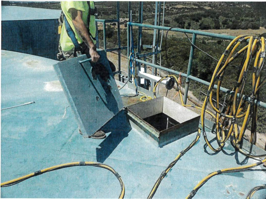
The photo above shows the roof hatch cover that is broken off.
