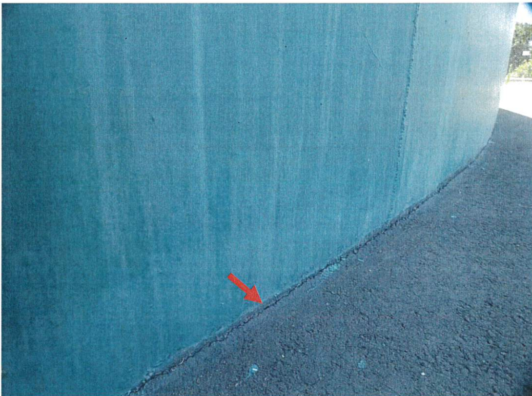
Another view of the lower shell. The arrow indicates a crack at the interface between the tank and the asphalt concrete paving. It appears that the paving does not seal out water but does prevent access for coating and inspection.
