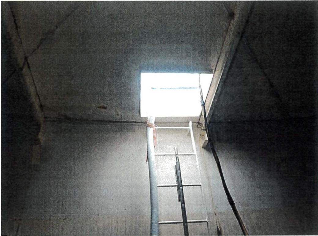
View of the roof hatch from the interior. The ladder is in good condition overall but some minor corrosion points are present.
