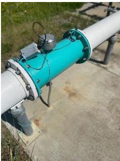
New Meter for Well #6:
